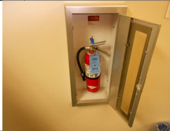
Photo #51: Fire extinguisher
