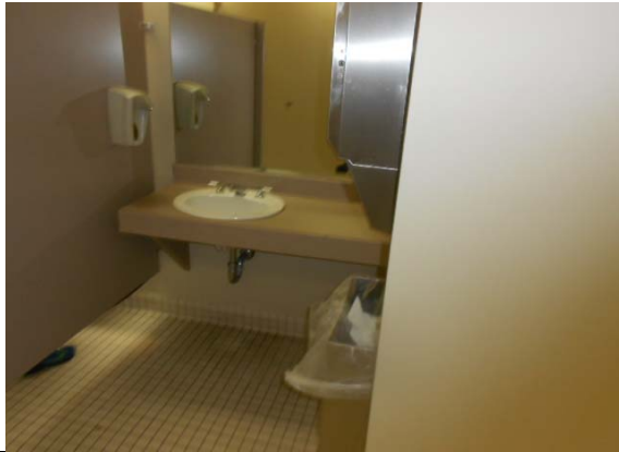
Photo #13: Common area restroom – Missing pipe insulation below sink
