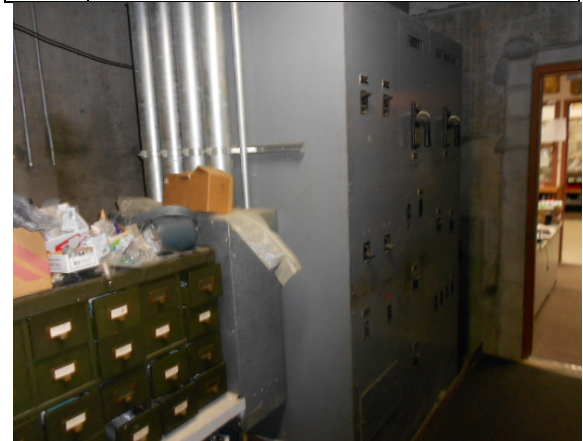
Photo #46: Main electric switchgear
