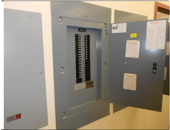
Photo #68: Tenant unit – Electrical panel
