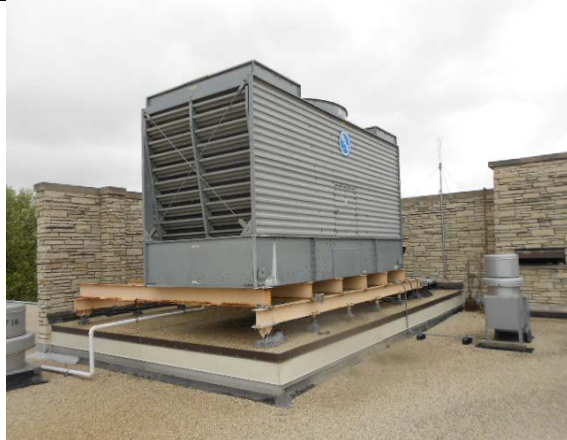
Photo #43: Cooling tower
