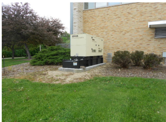
Photo #47: Emergency generator
