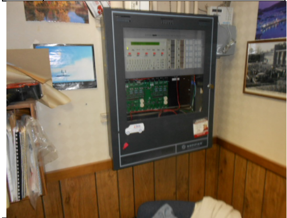
Photo #52: Fire alarm control panel
