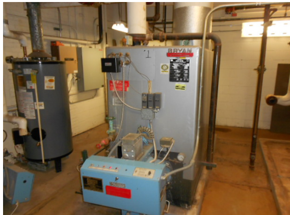
Photo #41: Heating boiler
