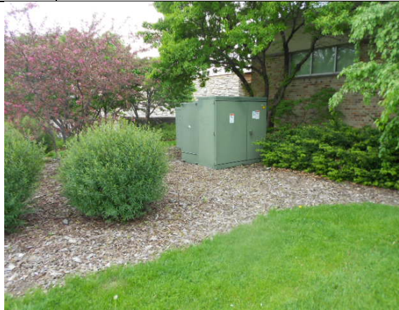
Photo #45: Pad mounted electrical transformer
