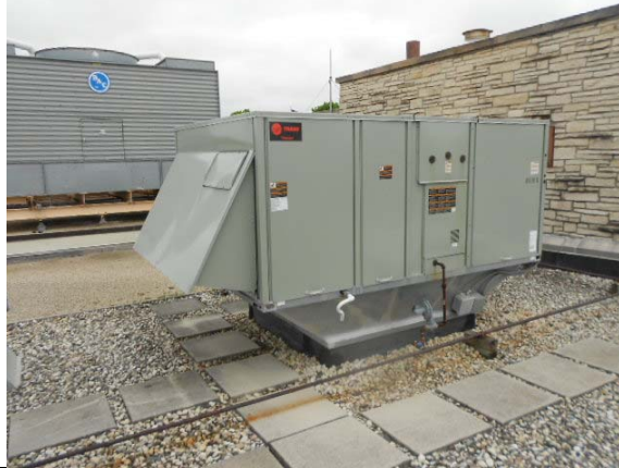
Photo #39: Rooftop HVAC package unit
