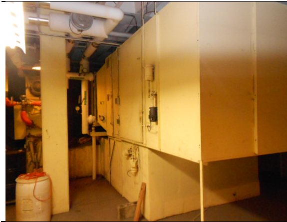
Photo #67: Air-handling unit
