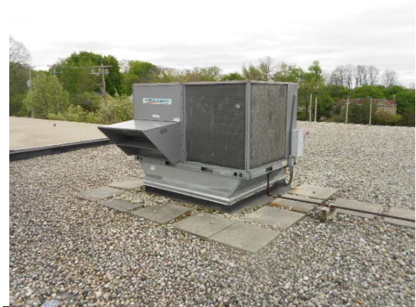
Photo #40: Rooftop HVAC package unit
