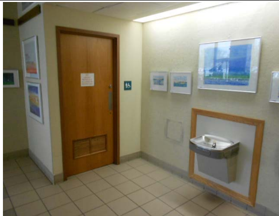
Photo #37: Drinking fountain
