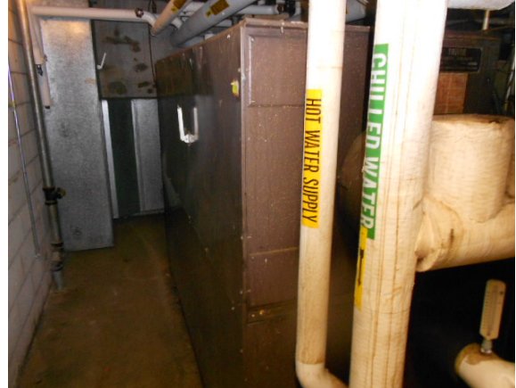
Photo #66: Air-handling unit
