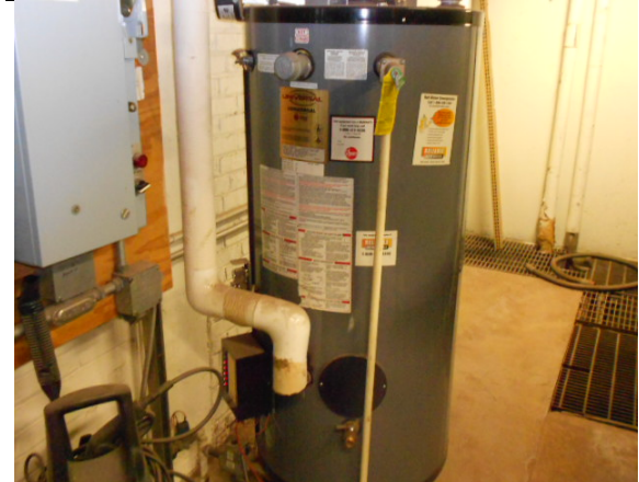
Photo #44: Domestic hot water heater (rented)
