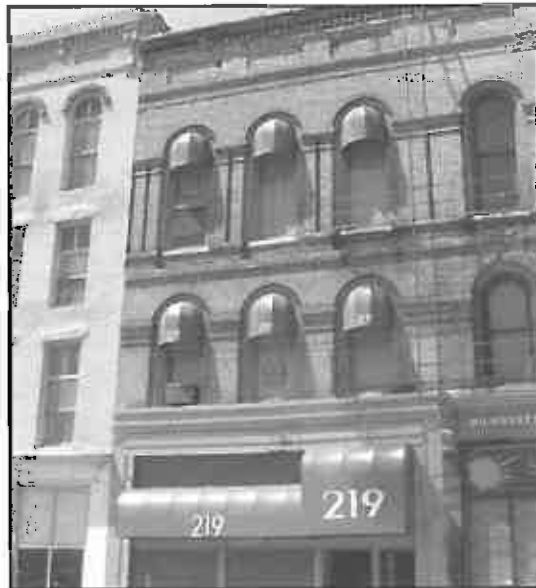
Inappropriate: Hard plastic awning in stiff framework; material does not compliment building.
