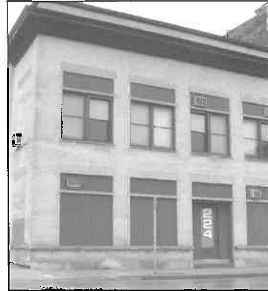
Inappropriate: Storefront windows completely filled in, top portion of upper window opening closed-in to accommodate new windows.
