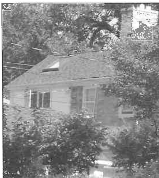
Appropriate: Skylight located on the rear elevation of the home. The unit is not visible from the facade or main street (9615 Harding Boulevard).
