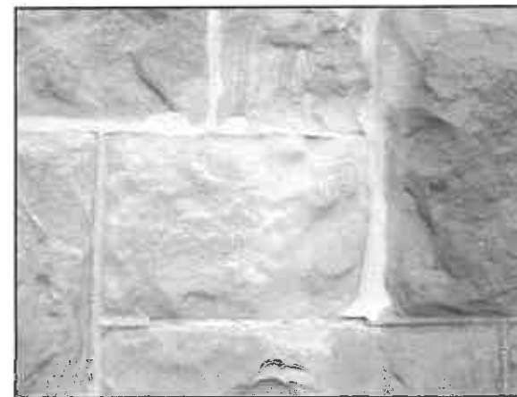
Inappropriate: Improperly repointed mortar joint, mortar covering face of stone unit.
