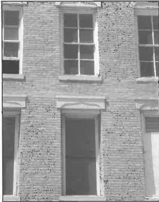
Inappropriate: Replacement windows do not match the material or 4-over-4 panel pattern of the original.
