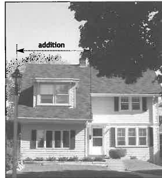
Inappropriate Facade Addition: This addition completely changes the appearance of the facade. Details such as window type and articulation do not match the existing home.
