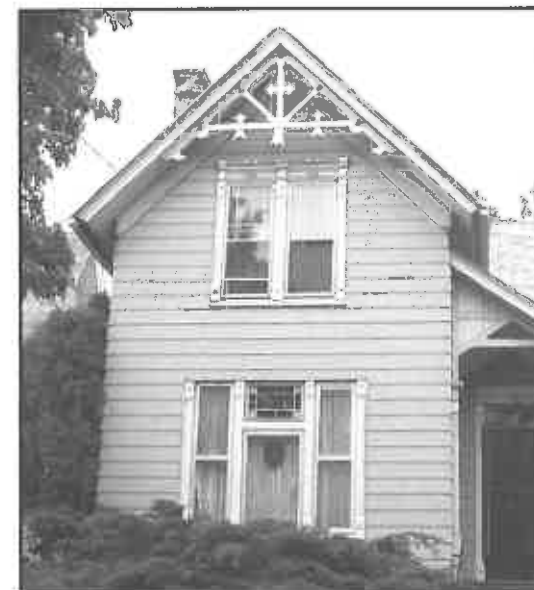
Inappropriate: Aluminum siding covering clapboards.
