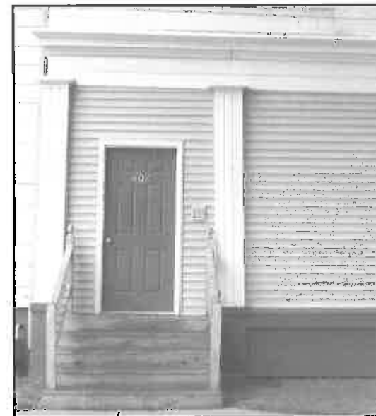
Inappropriate: The completely enclosing of an open porch shall not be permitted. Steps and railing are inappropriate materials and detailing
