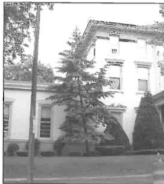
Inappropriate Side Elevation Addition: The detailing and materials of this addition are similar to that of the existing home. However, the scale and massing are so out of character with the existing home that it is distracting.
