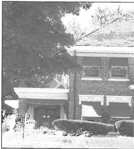
Inappropriate Side Elevation Addition: This small addition is not in keeping with the style, character, window articulation or detailing of the original home.
