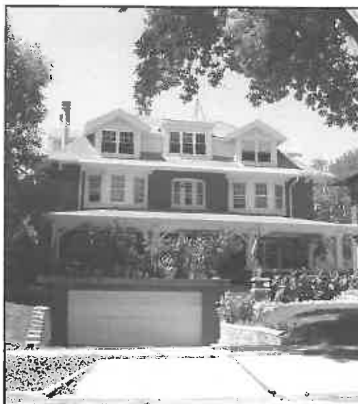
Inappropriate Garage Addition: This garage detracts from the facade elevation, disrupts the setting and obscures the view of the porch.
