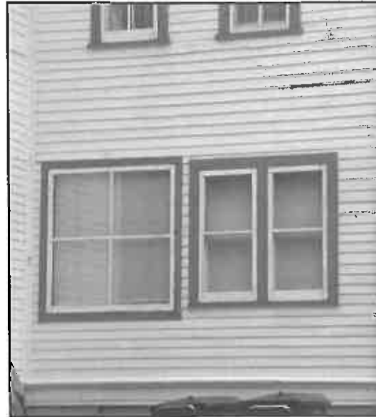
Inappropriate: New window larger than existing unit.
