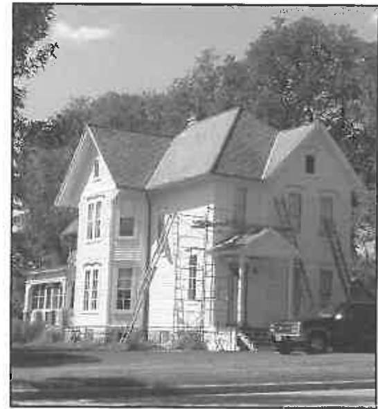
Maintenance and repair in action: Asphalt shingle siding was removed to reveal clapboard siding (12231 Watertown Plank Road).
