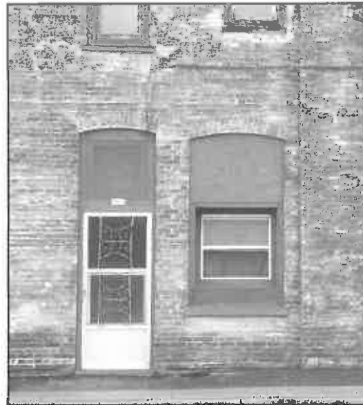
Inappropriate: Original window opening filled with wood to accommodate smaller vinyl replacement unit.
