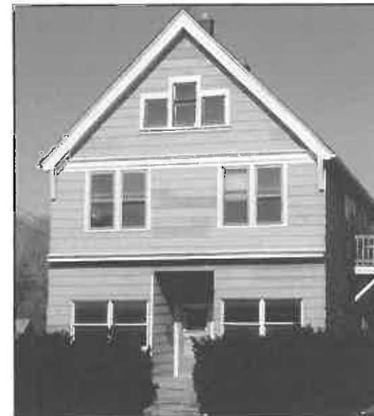
Inappropriate: Aluminum siding covering wood shingles.
