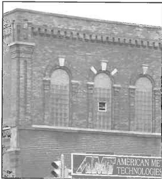
Inappropriate: Original window opening infilled with glass block and wood.
