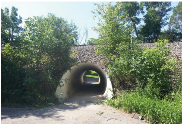
Existing tunnel at Hansen Golf Course is too short for bicycle users.
