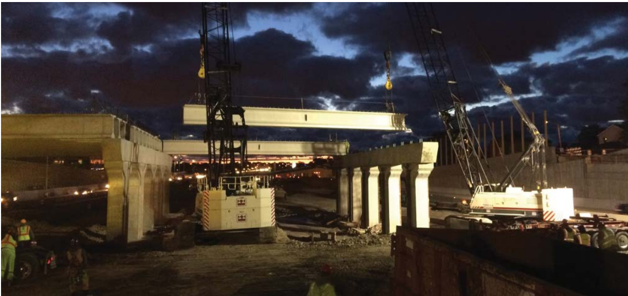
The Wisconsin Zoo Interchange Project is a large-scale infrastructure upgrade targeted at alleviating traffic congestion. The 92nd Street bridge is rebuilt in the photo above. Source: WisDOT
