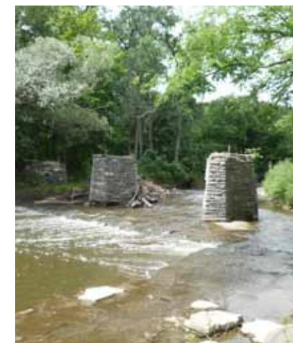
Bridge Piers. These structures could be used to support a trail bridge to link the River Parkway corridor with Honey Creek Parkway and Jacobus Park.
